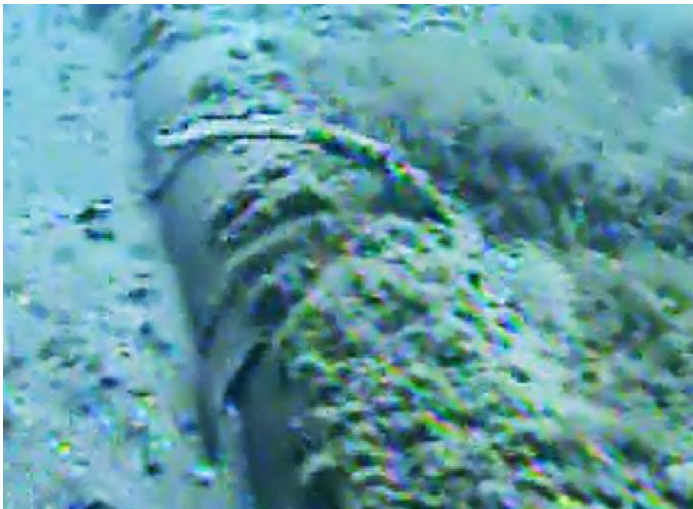
Figure 10. Detail from Photo Clipped from Enbridge 2012 Underwater Inspection Video of the West Line Taken on 8/25/2012 at 15:58:44 Showing Disbonded Coating and Broken Band
