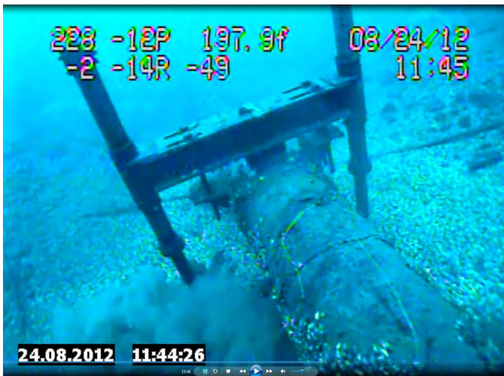
Figure 8. Photo Clipped from Enbridge 2012 Underwater Inspection Video of the East Line Taken on 8/24/2012 at 11:44:26 Showing Missing and Disbonded Coating
