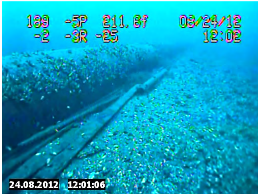
Figure 6. Photo Clipped from Enbridge 2012 Underwater Inspection Video of the West Line Taken on 8/24/2012 at 12:01:06 Showing Detached Slats.
