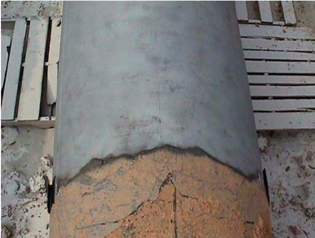
Figure 12. Typical Corrosion Found Under a Disbonded Coating as Reveled by Light Abrasive Blasting
