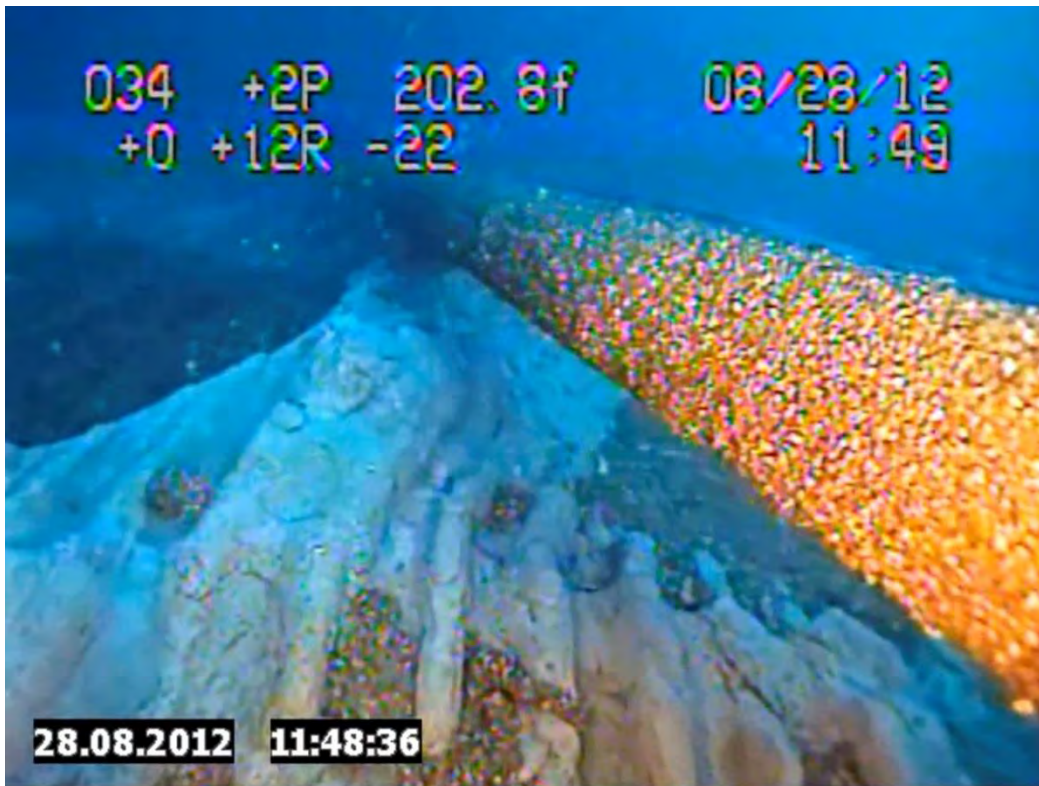
Figure 19. Photo of Unsupported Span Clipped from Enbridge Underwater Inspection Video from the 2012 Inspection (East Leg, ~203 feet water depth)
