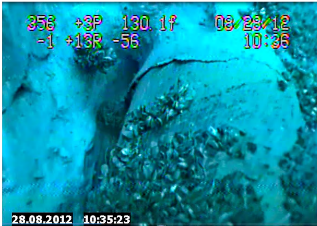
Figure 7. Photo Clipped from Enbridge 2012 Underwater Inspection Video of the East Line Taken on 8/28/2012 at 10:35:23 Showing Missing and Disbonded Coating
