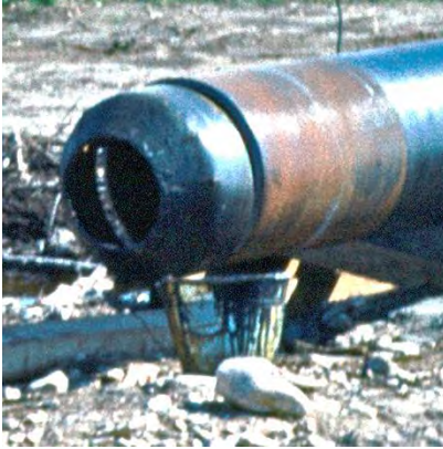
Figure 3. Detail Enlarged from Trudgen Photo of Pipe Wrapping Machine Showing Wrapped Pipe (00010370012.tif)
