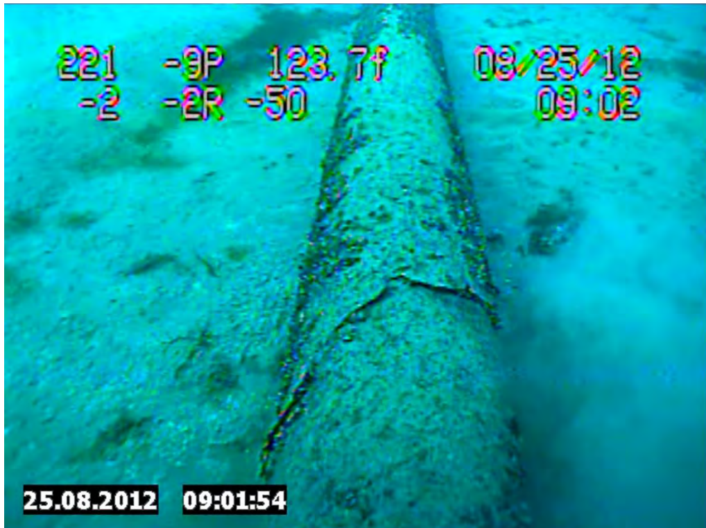
Figure 9. Photo Clipped from Enbridge 2012 Underwater Inspection Video of the East Line Taken on 8/25/2012 at 09:01:54 Showing Missing and Disbonded Coating
